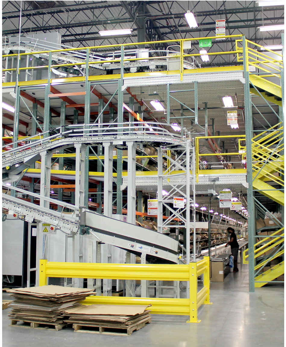
The three-level piece pick module is configured with a zone route conveyor network.
