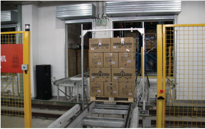
Pallet profile checking prior to ASRS.
