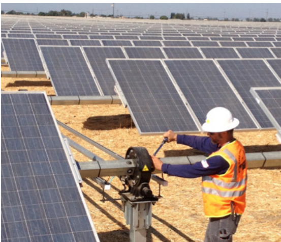
Expertise in installing and maintaining utility-scale solar (also known as solar parks or solar farms)
